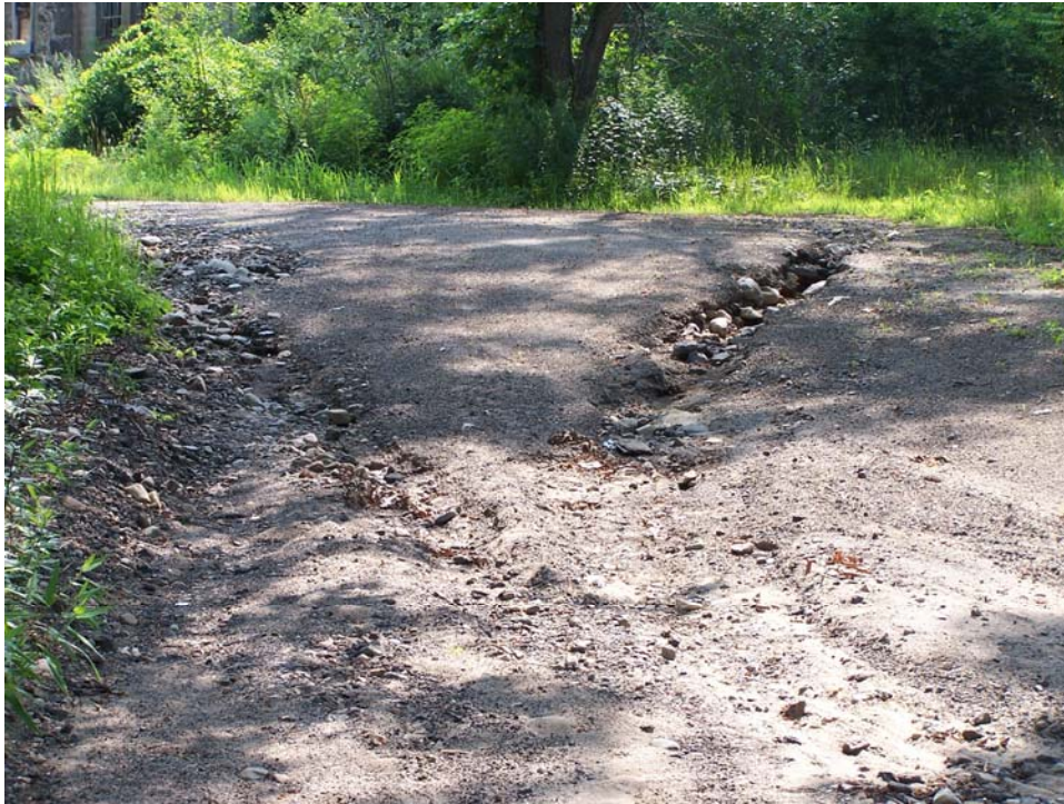
Figure 2. Dirt Road eroding into river at Bridgewater Highway Dept
