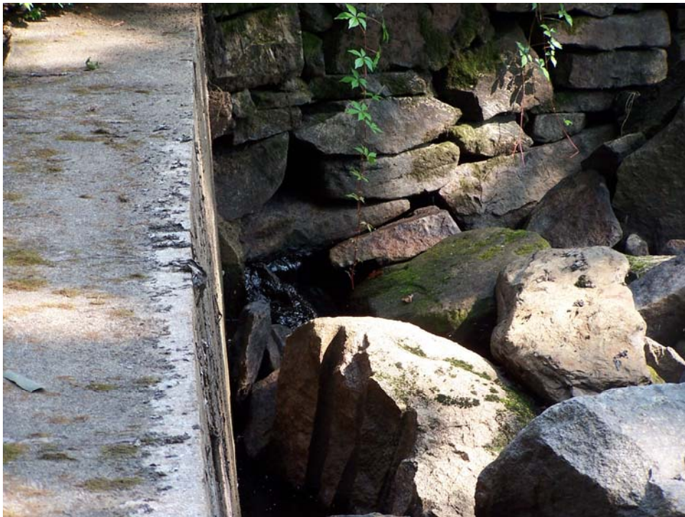
Figure 4. Seepage through War Memorial Dam
